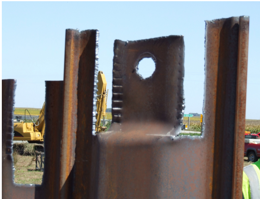
Figure A.5. Buckled sheet pile section due to driving equipment.
