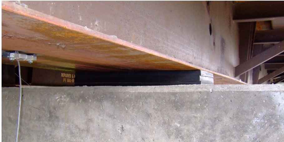
a. 1-inch Neoprene Bearing Pad under Interior Girder at Pier
