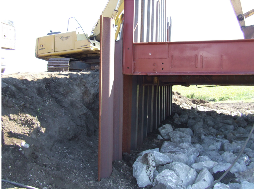
Figure A.4. Sheet pile abutment construction with no expansion joint provided.
